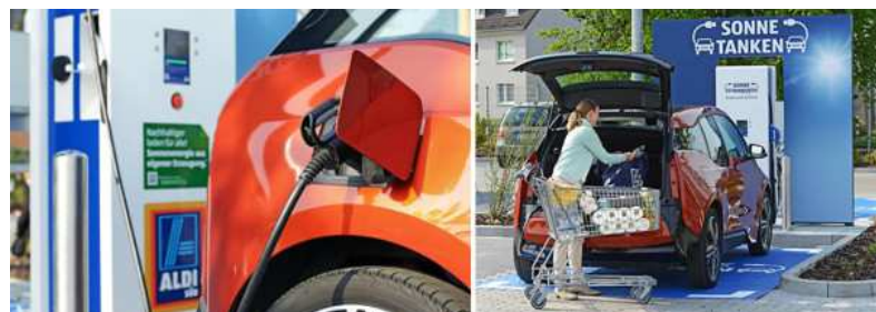
Germany's Aldi supermarkets is installing Efacec QC20 DC fast chargers at 50 stores in Dusseldorf (shown here), Frankfurt, Cologne, Mülheim an der Ruhr, Munich and Stuttgart.
